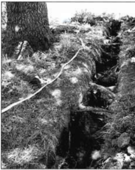
Pneumatic or hydraulic tools can be used to remove soil around tree roots to determine their number and size, to expose them so they can be cut with a saw, or to thread pipes or conduit under them rather than cutting.
